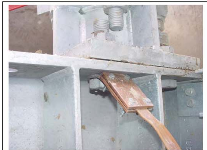
Grounding connection point to the tower leg
