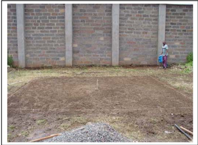
Once the exact difference between the 4 corners of the lot is known. The 4 corners are marked and a rope is set at a level
