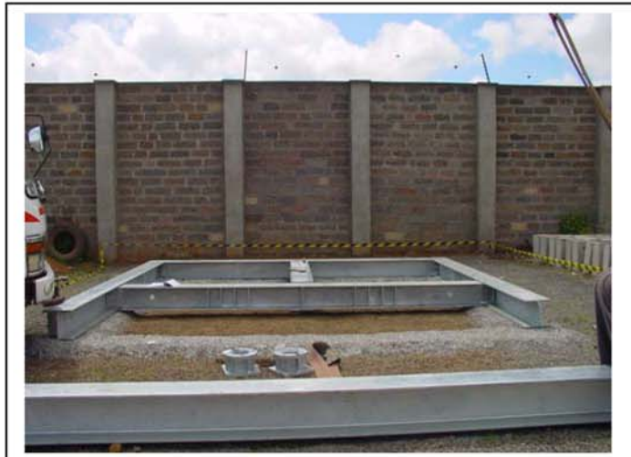
Beams P1 and P5 placed on location Levels are verified prior continuing with the next step
