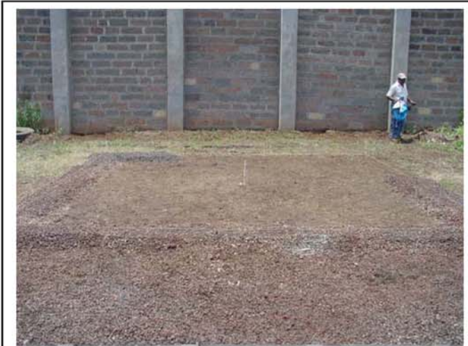
Gravel ½ inch is used in order to achieve an exact leveled area. This is places in a form of a square around the 4 corners
