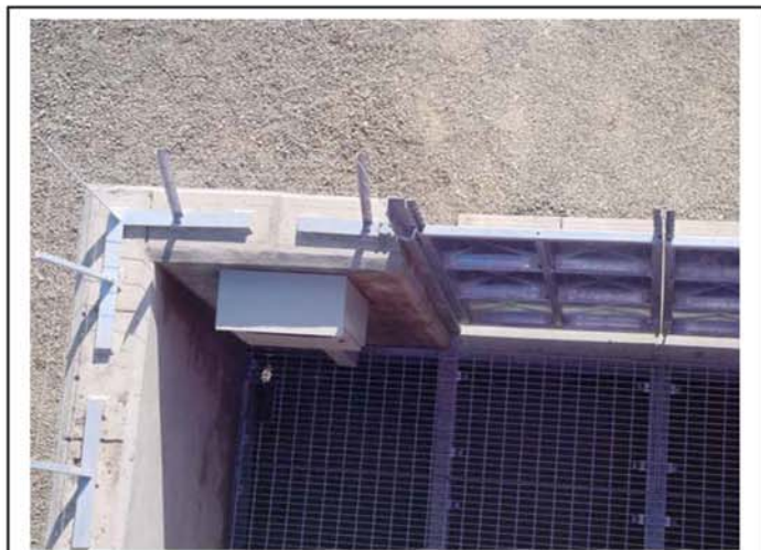
View of energy meter box
