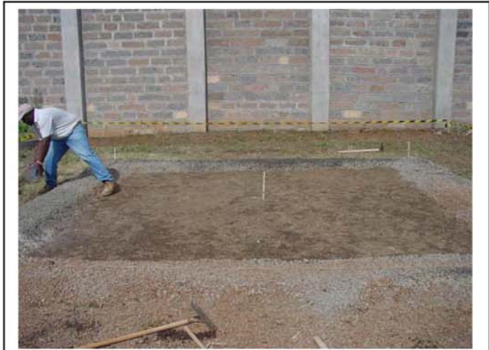
A mix of cement and water is purred on top of the leveled gravel. This is intended to keep the gravel in place during installation
