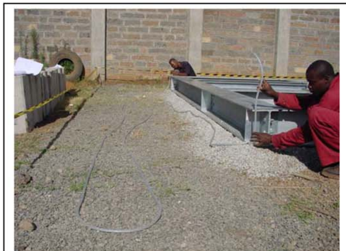
By using a Water pipe as level, we make sure that the completed structure is leveled
