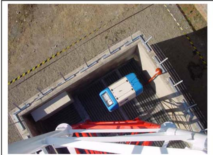
Generator and electrical cabinet from tower
