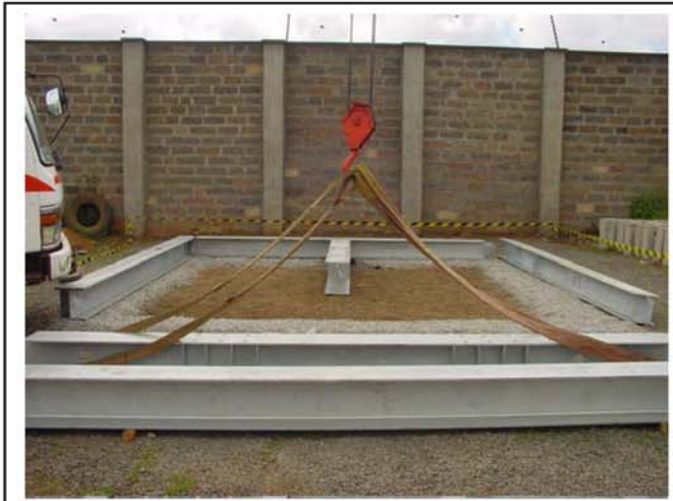
Beam P2 is placed on location – (P5 aside) Levels are verified prior continuing with the next step
