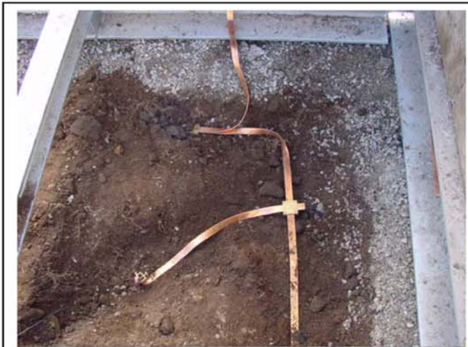
Grounding installation according to the specified design – Copper tape and rods are installed
