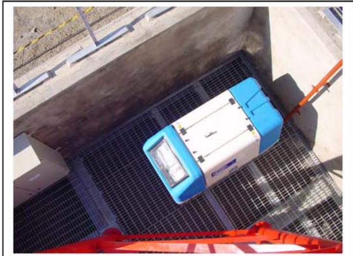
Generator from top for Tower
