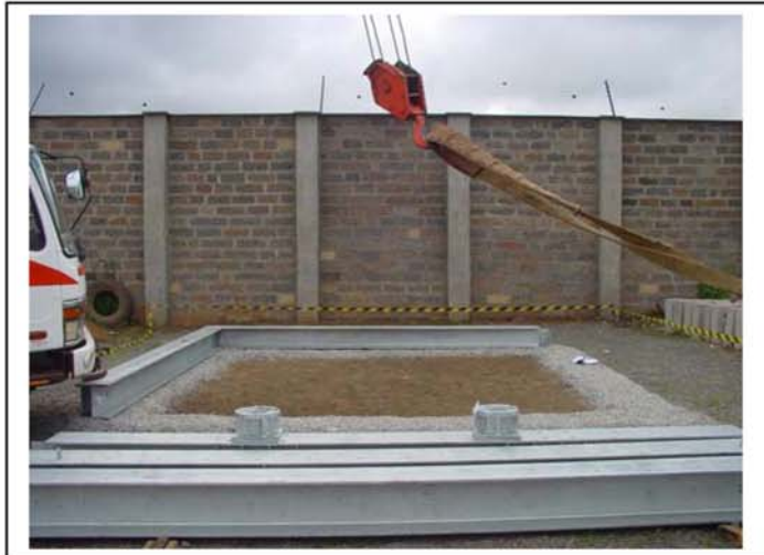
Beam P3 is placed on location. Levels are verified prior continuing with the next step
