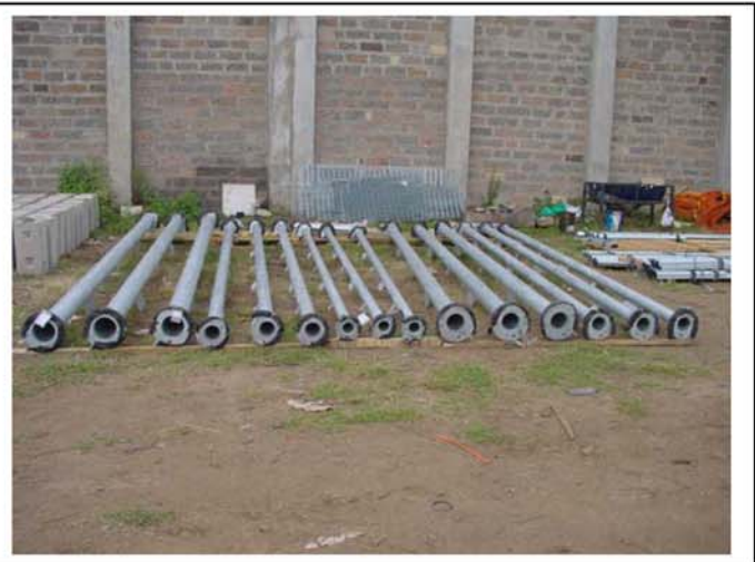
Tower main legs
