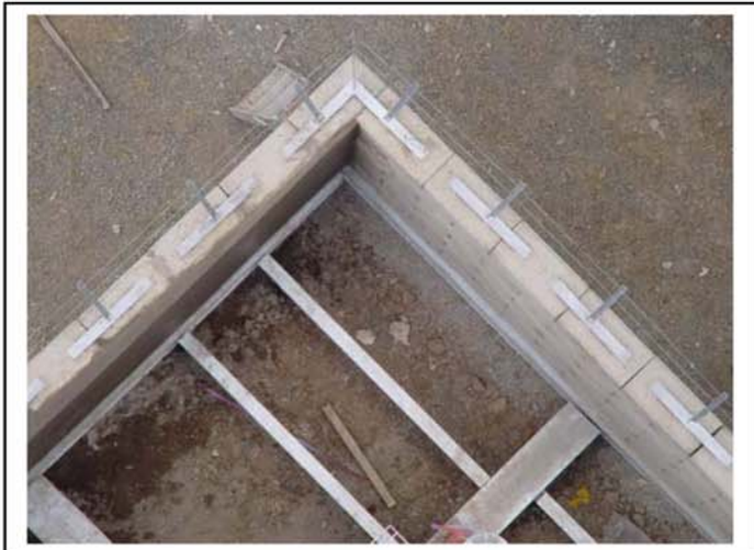
Installation of the Steel Wire as a preparation for future installation of Razor Wire
