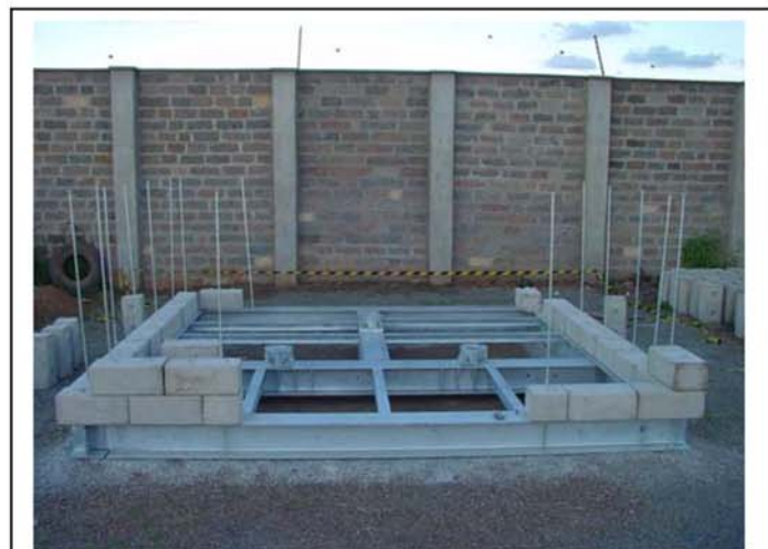
Startup with the placement of the blocks – The Rods are continuously inserted to make sure the blocks are in Place
