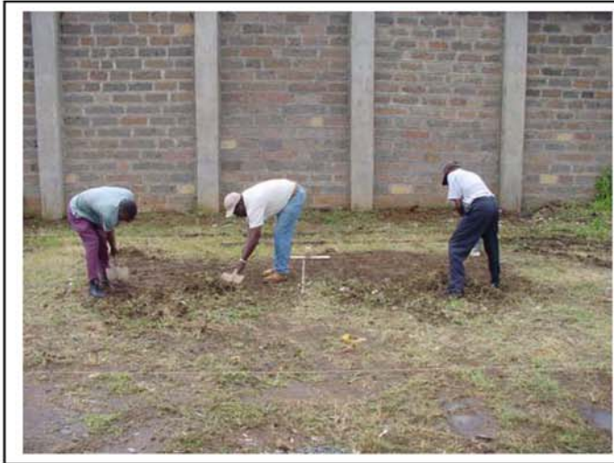
6m 2 of land is being cleared to accommodate the QS frame. This area is nearly leveled at all side but still need minor adjustments
