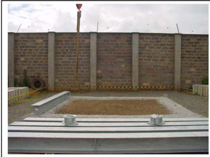
Beam P4 is placed on location Levels are verified prior continuing with the next step
