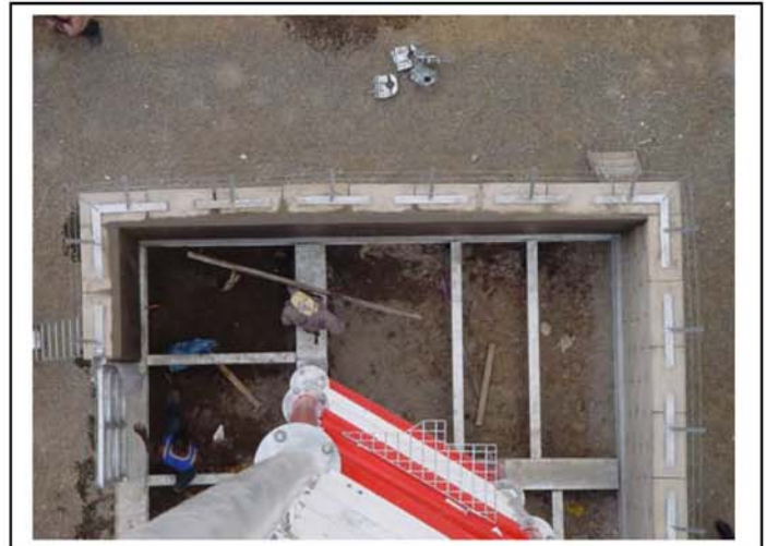
Installation of the Steel Wire as a preparation for future installation of Razor Wire
